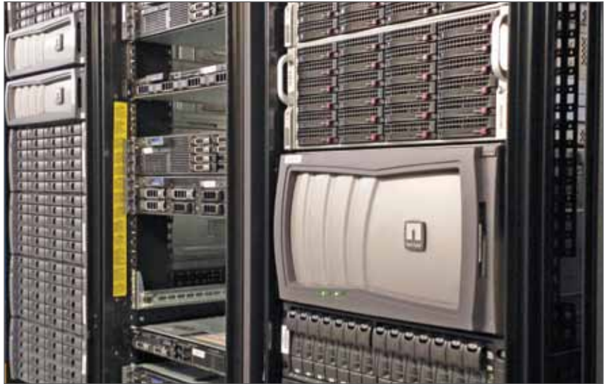
Figure 1-5. JHC/CCOM SAN and NAS infrastructure in the primary server room.
