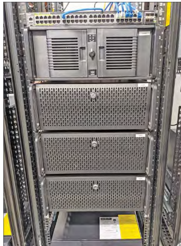
Figure I-8. Custom GPU compute cluster in its rack, installed in 2020.
