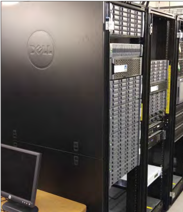
Figure I-7. Center SAN and NAS infrastructure in the primary server room.
