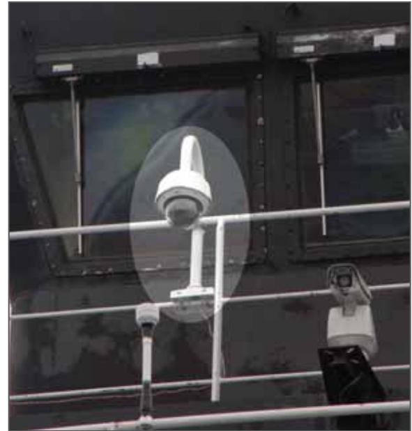
Figure 7-10. The geoCamera v2.0 installed outside the Aloft-Con on the USCGC Healy .
