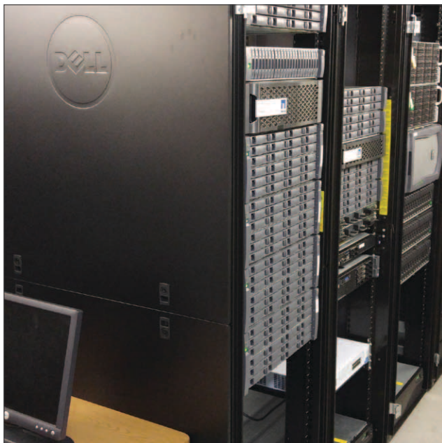
Figure I-8. Center SAN and NAS infrastructure in the primary server room.
