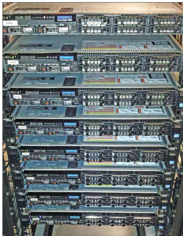
Figure I-8. Dell computer cluster in its rack.
