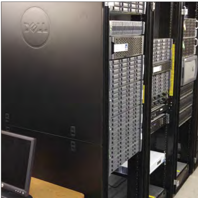
Figure I-7. Center SAN and NAS infrastructure in the primary server room.
