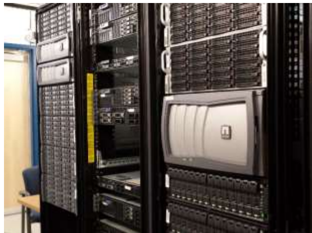
Figure 1-5. Center SAN and NAS infrastructure in the primary server room.
