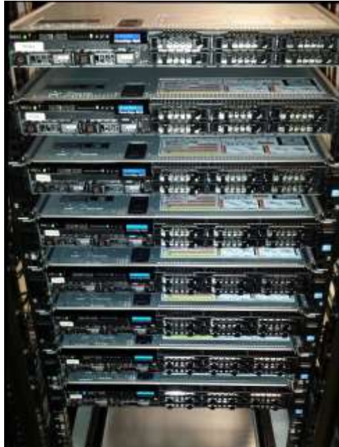
Figure 1-6. Dell computer cluster in its rack, installed in 2014.
