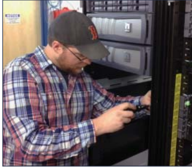
Will Fessenden installs rack rails for the new storage area network (SAN).
