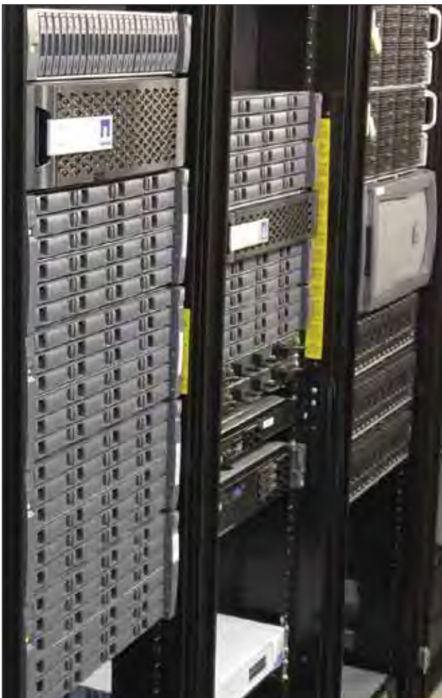
Figure 1-7. Center SAN and NAS infrastructure in the primary server room.
